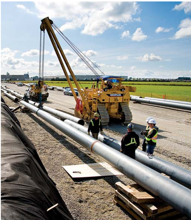
The approximate $27 million Fraser River South Bank South Arm Rehabilitation Project is expected to be in service by the end of August 2010.
