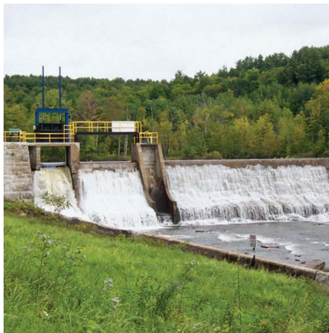
Fortis Generation has a combined generating capacity of 139 MW, 134 MW of which is hydroelectric generation.
